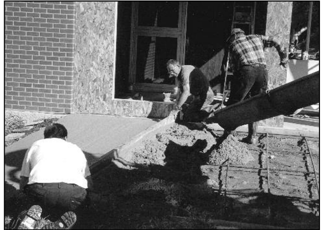
Brother Randy, Al Vedress and Brother Basil working on the cement pad at the entrance to the renovated abbey elevator.
