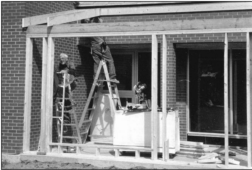
Brother Wolfgang on the ladder and Alan Vedress framing the new entrance to the church elevator entrance.
