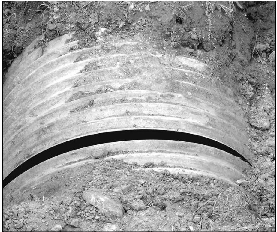
This culvert on the abbey road to Muenster came apart on a seam during this spring's runoff.
