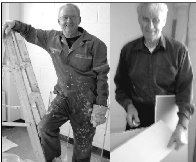
Much retrofitting in abbey rooms is underway. Two of Abbot Peter's brothers, Arnie Novecosky (left) and Leonard Novecosky (right), helped carpenter Br. Wolfgang.
