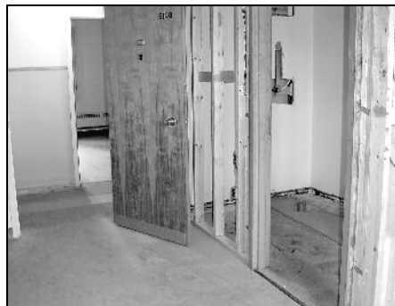
Basement of Severin Hall is being remodeled into individual boarding rooms, mainly for foreign university students.
